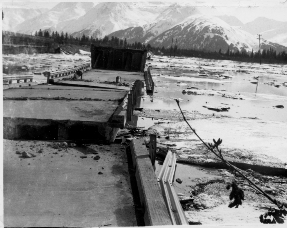
Photo Taken from 1st Span Looking Down at 20 Mile River Bridge Going into Portage - Mile 20
